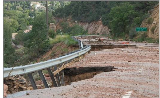
A road is severely damaged by flooding in Manitou Spring, Colorado, 2013.
